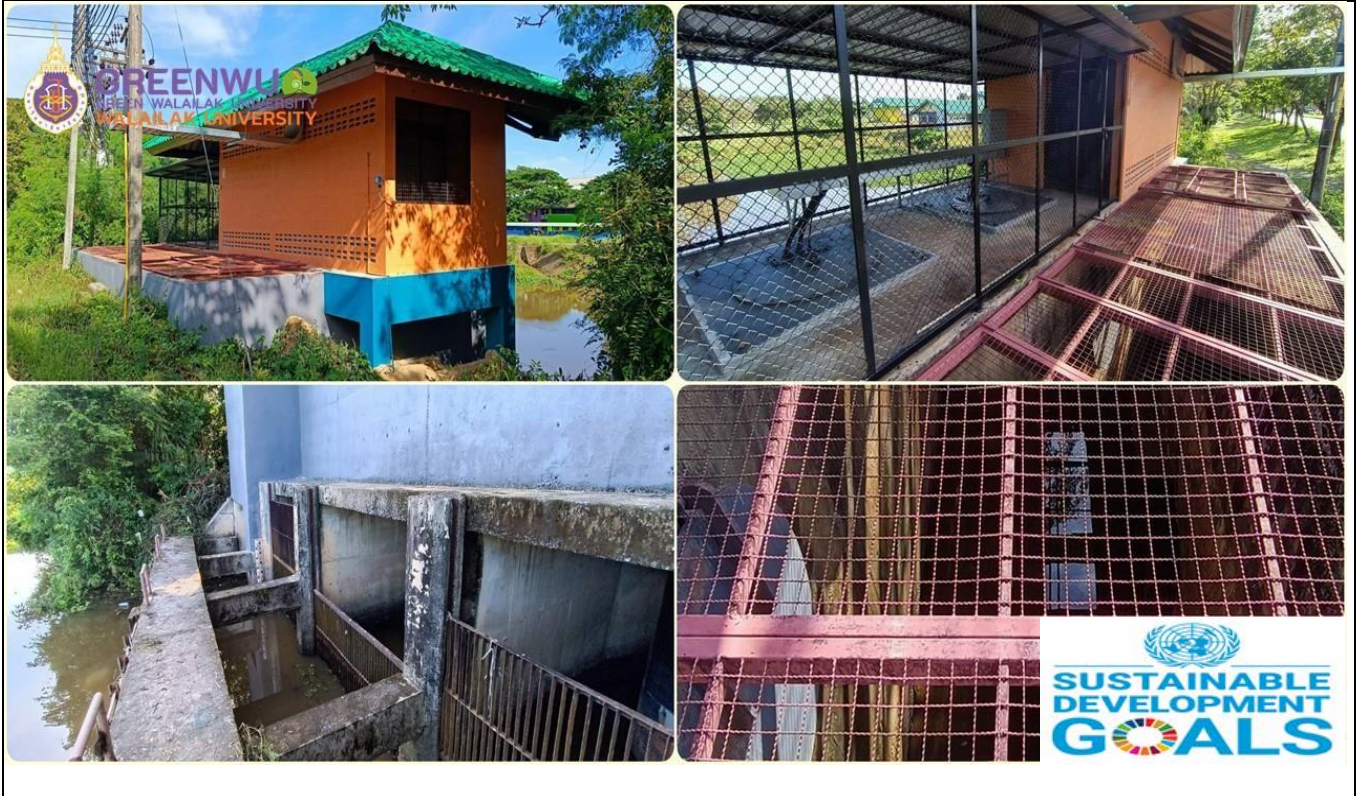
6.3.3-12 Water pump in case of flooding (Walailak University, Thailand)
